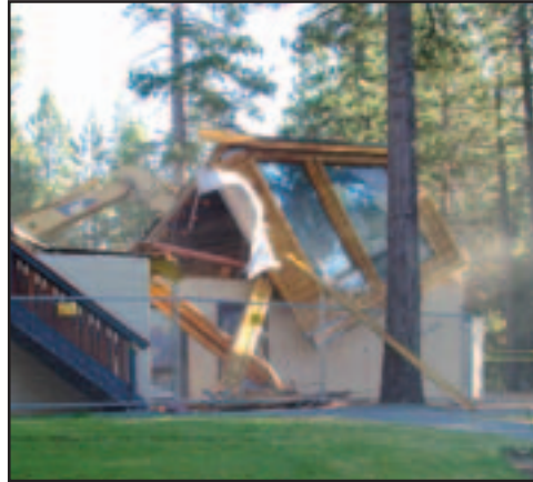
The old golf course clubhouse was demolished on October 20 to make ready the site for construction next spring. Photos by Dana Gravelle
